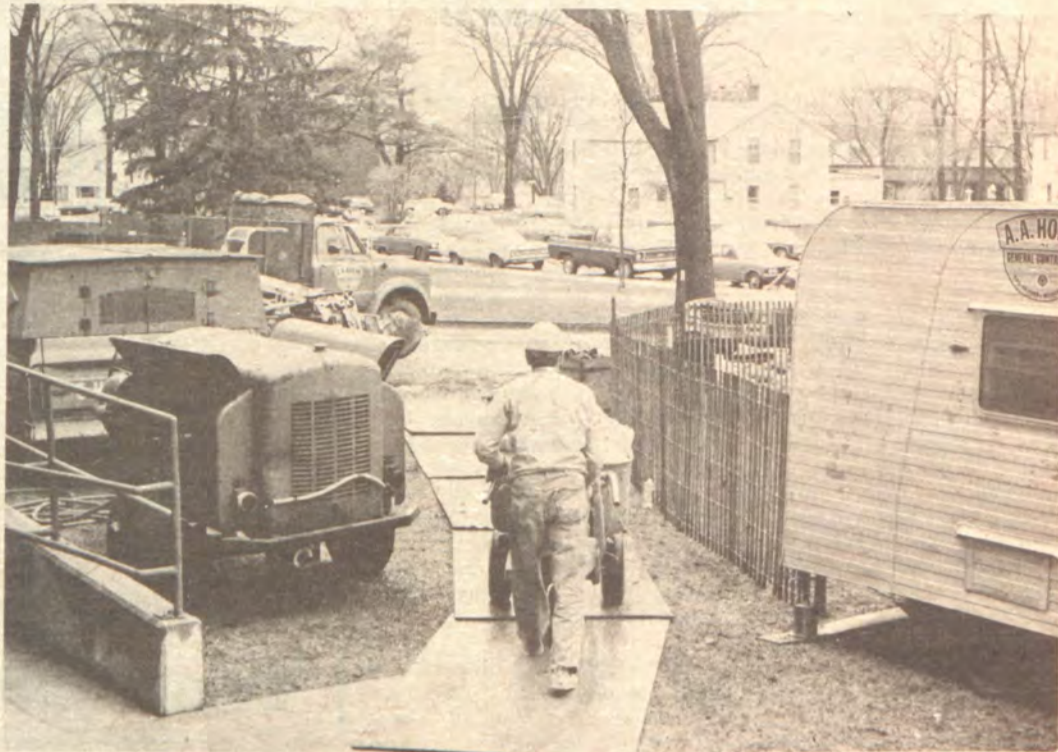
The Spring Street side of North Hall bears most of the construction traffic. Photo by Sue Hausman
