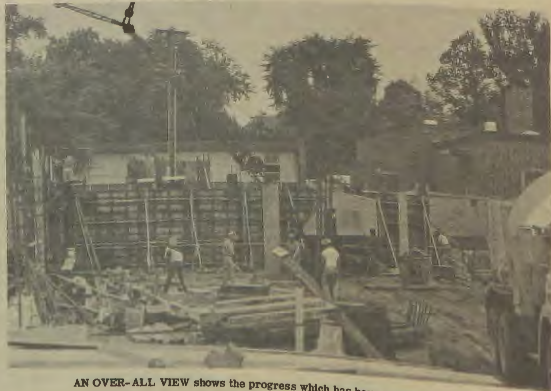
CONSTRUCTION CONTINUES on the new addition to the Student Center. Here workmen pour concrete for one of the foundation walls.
