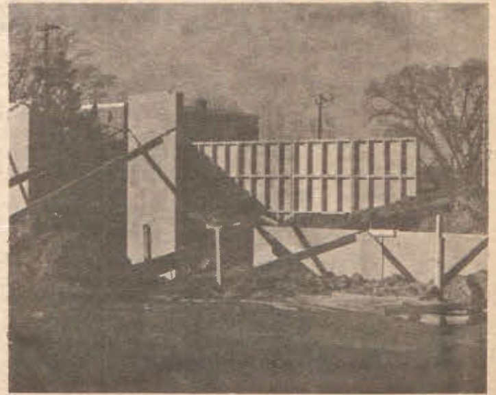
CONSTRUCTION OF HARDEE'S brings charcoal broiled burgers closer to UW-RF. Photo by Pat Hildebrant.
