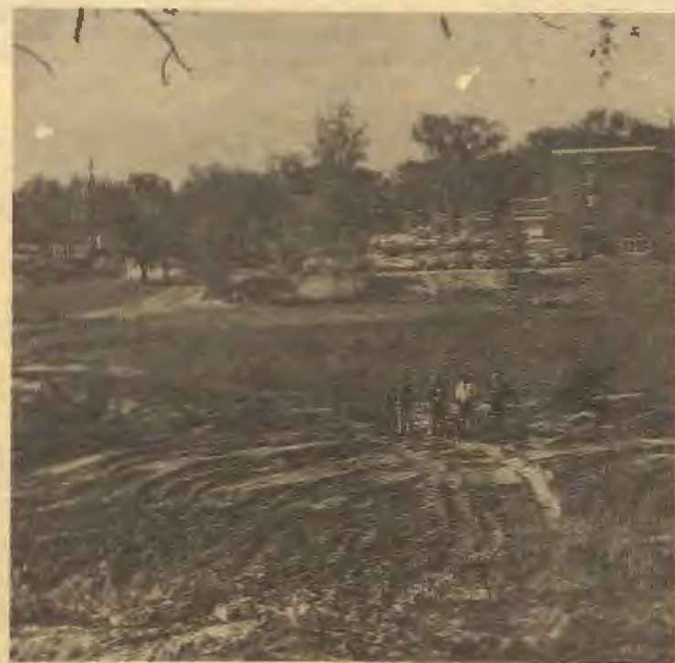
CHECKING THE PROGRESS of the Amphitheatre being constructed along the South Fork Creek area are, left to right, George Wirth, an oldtimer from River Falls, and Foundation Committee members Harvey Stower, Bob MacGregor, and Dr. Melvin Wall.
