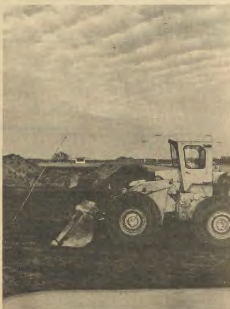
Work on the $895,000 All-Purpose Arena started recently near Ramer Field. Assistant to the Chancellor Wilbur Sperling said that excavation will begin May 1 with completion set for one year from that date (May 1973). General contractor is Gunnar Johnson, Minneapolis. Jim Francois photo.
