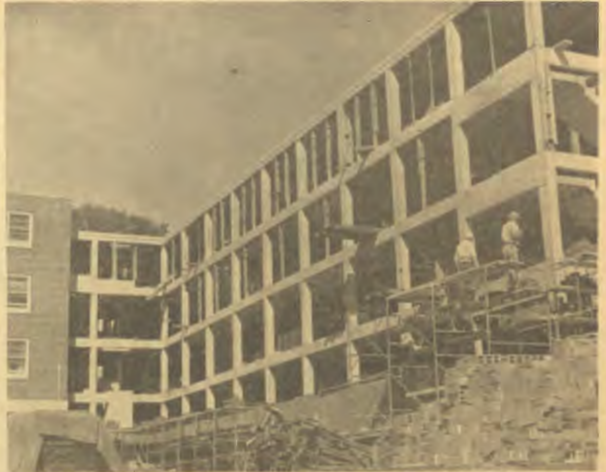
Loes and workmen depict the present stature of the new wing being added to Hathorn Hall as the new structure rapidly climbs and develops under the eyes and skills of engineers, architects and skilled workmen. The new wing is expected to be livable by the fall of 1962 housing 142. It is intended to relieve some of the pressure of overcrowding that now exists in women's housing.
