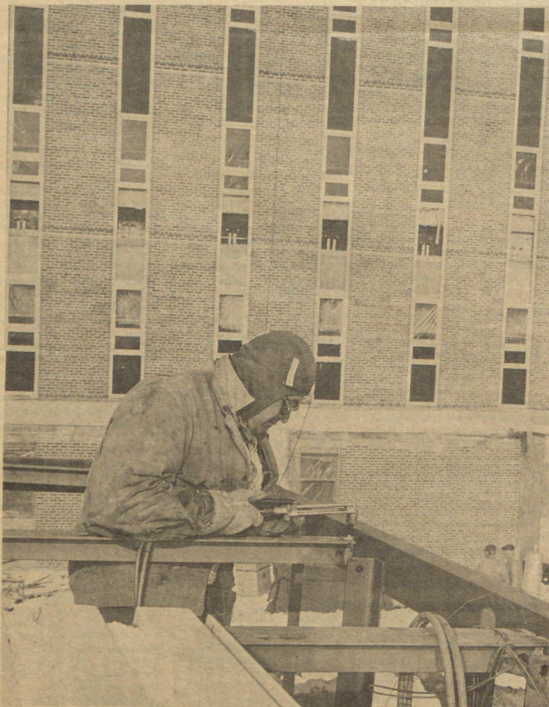
A WELDER BRAVES the cold as he joins building. Behind him is a portion of the four-story structure. (Voice Photo).
