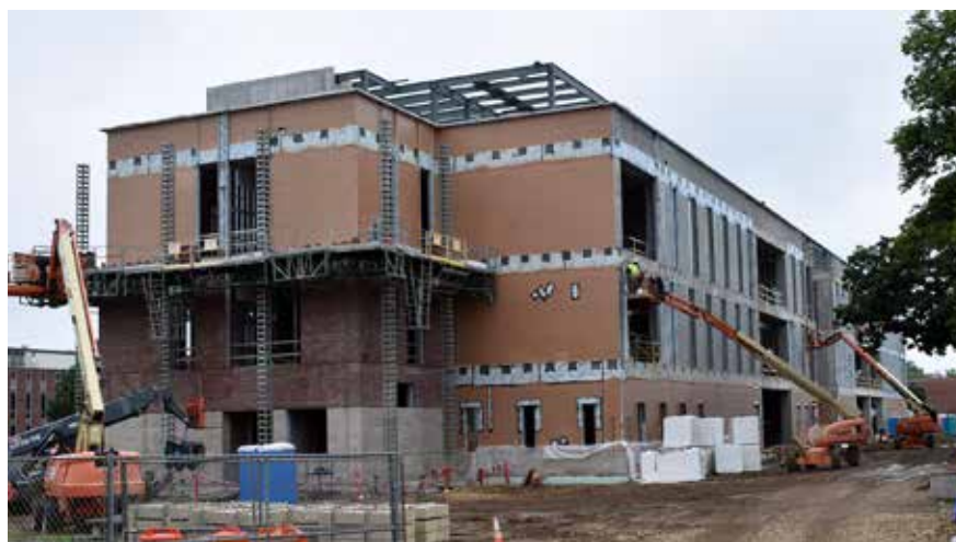
A view of the northeast corner of the SciTech building, taken on July 2. The Physics department will occupy the first and second floors of the east side of the building. The windows on the north east corner of the first floor shown here are where the Advanced Lab will be located, and directly above that will be the Astrophysics lab.
