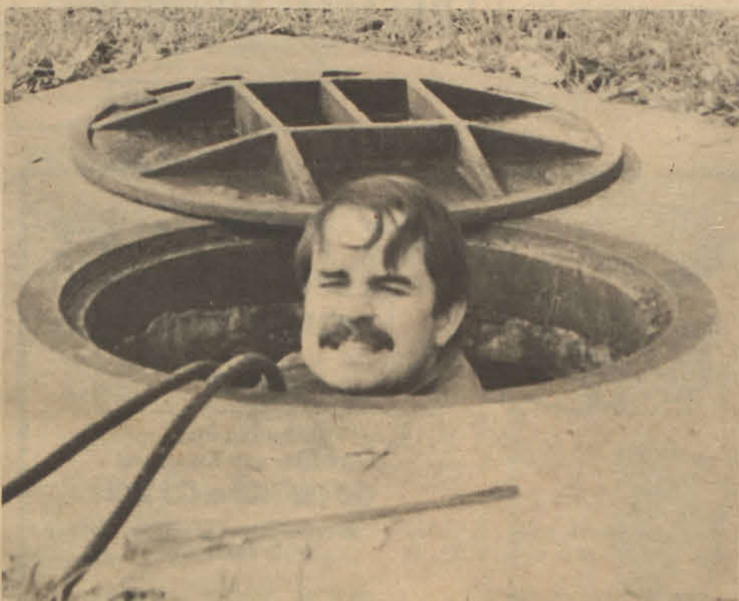
GETTING READY for a long winter hibernation. UW-River Falls' Mr. Fix-it, Al Murray, is doing some electrical work
