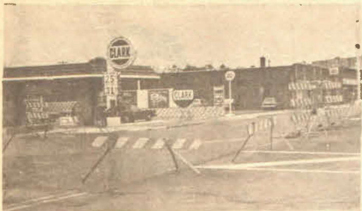
Downtown construction has stepped up traffic through town. Photo by Mary Meysembourg.
