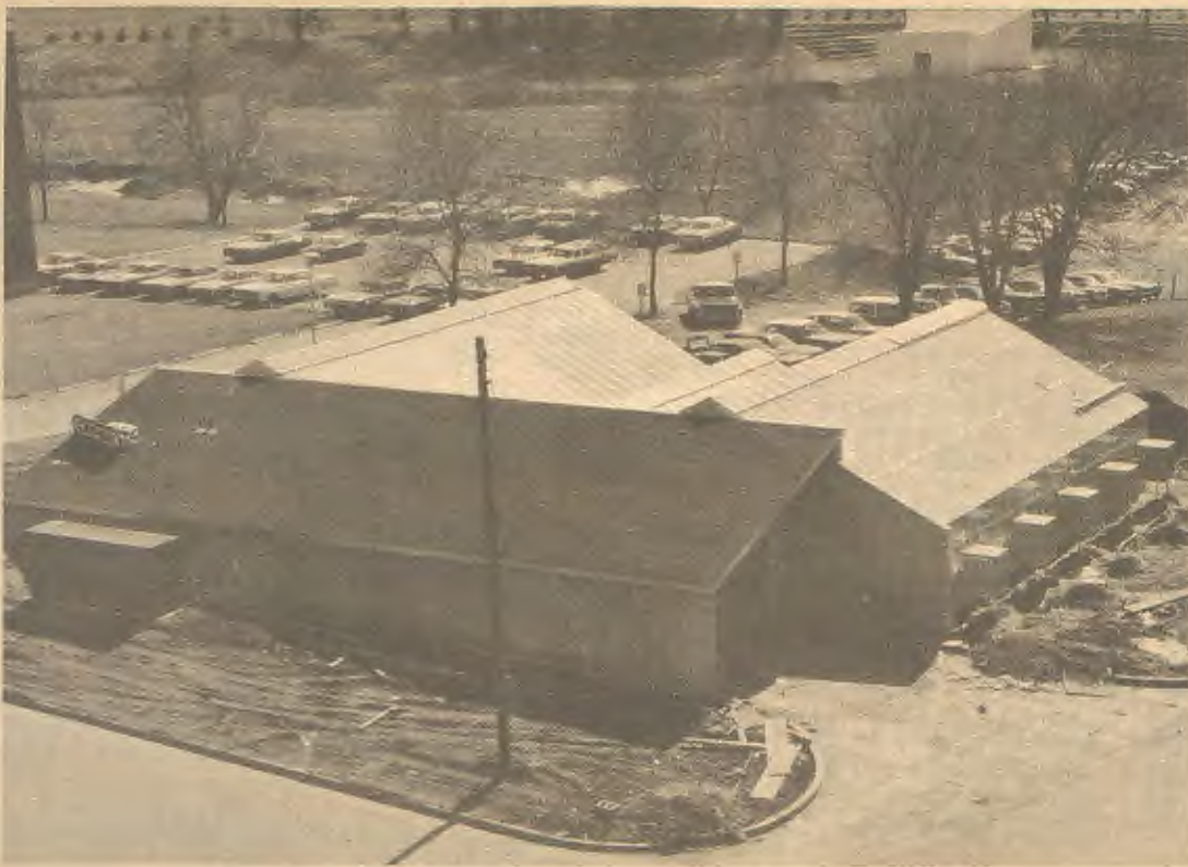
View of the new greenhouse now under construction behind Ag. Science. (Oftedahl photo)
