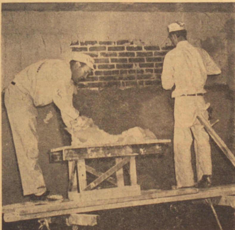
Plasterers are busy at work applying the primary coat to the interior walls of the soon-to-be-completed Chalmer Davee library on the campus.
