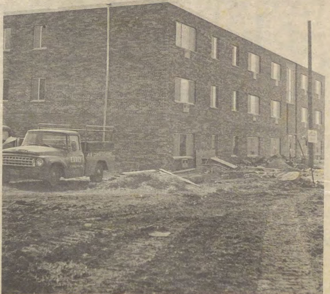
THIS NEW 33 UNIT APARTMENT BUILDING will be ready for occupancy in June. The new apartment building is located at 218 Charlotte St. The apartment building was constructed by Lowery Hill. They are also building another apartment house at the end of Cascade St.
