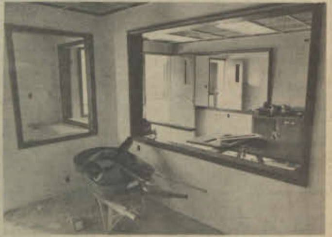
ITS STILL A LONG WALK before "Step 3," or any other program will be broadcast out of WRFW's new studio the new station, located in the third floor of North Hall, replaces an older facility that had its home in the North Hall basement. Construction will be completed in October. Photo by Randy Johnson.
