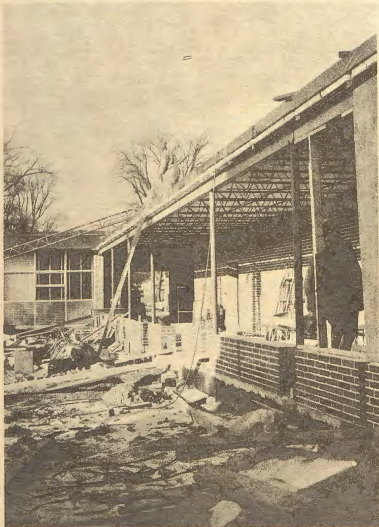
CONSTRUCTION PROGRESSES ON STUDENT CENTER ADDITION. (Looking north toward east end of Karges Center.)
