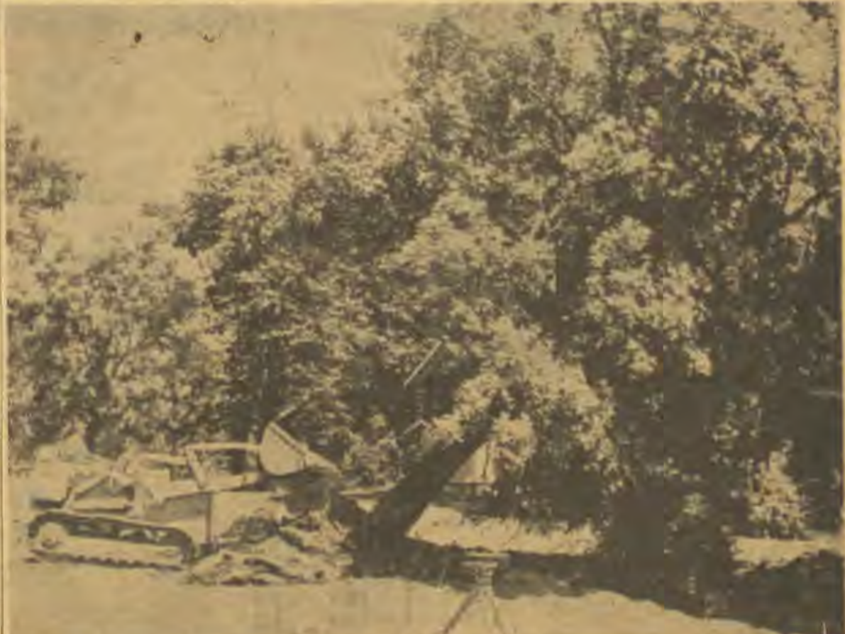
THIS LARGE OAK TREE on the River Falls State College campus gave way to progress this summer as workmen began construction of a wing on Hathorn Hall, the women's dormitory. The dormitory wing was one of two major projects started during the summer.
