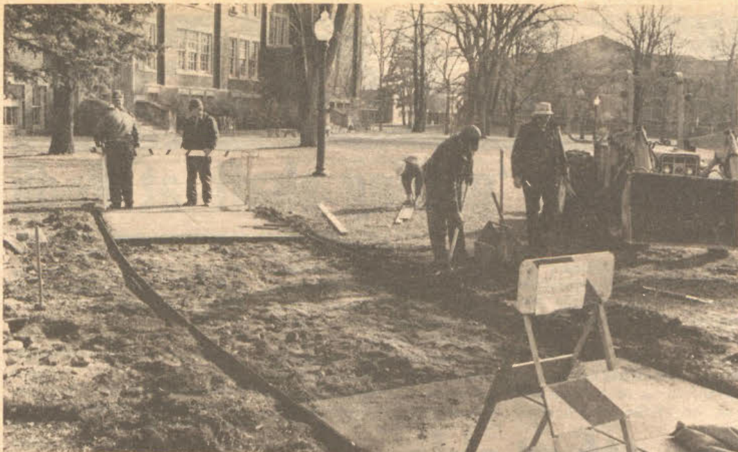
AS WORKERS RUSH TO FINISH BEFORE THE SNOW FLIES, this North Hall sidewalk gets resurfaced now by
