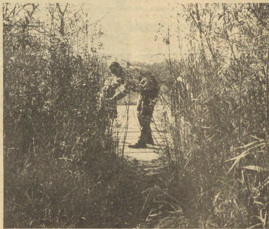
Editorial Board Director Mike Norman inspects peeling paint on a wooden bridge he "discovered" near the amphitheater. The bridge spans the South Fork in an area, if properly developed, could make WSU-RF one of the most scenic of the state universities.
