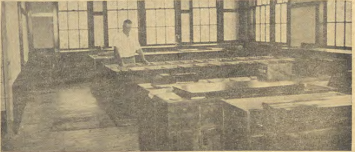
Room in which new chemistry equipment will be installed. The photo shows some of the new desks in which laboratory sinks and plumbing will be installed. Chemistry Instructor Setterquist is surveying his new domain.
