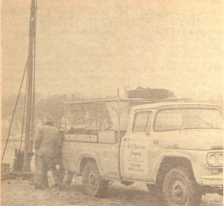
Workmen made test borings of the earth where the new addition to the Student Center will stand, last Monday.
