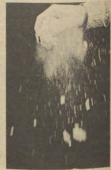
The spray fireproofing is a flakey, powdery substance and falls easily from the ceiling. Under the slightest pressure, it pulverizes into tiny particles which are invisible in the air.
