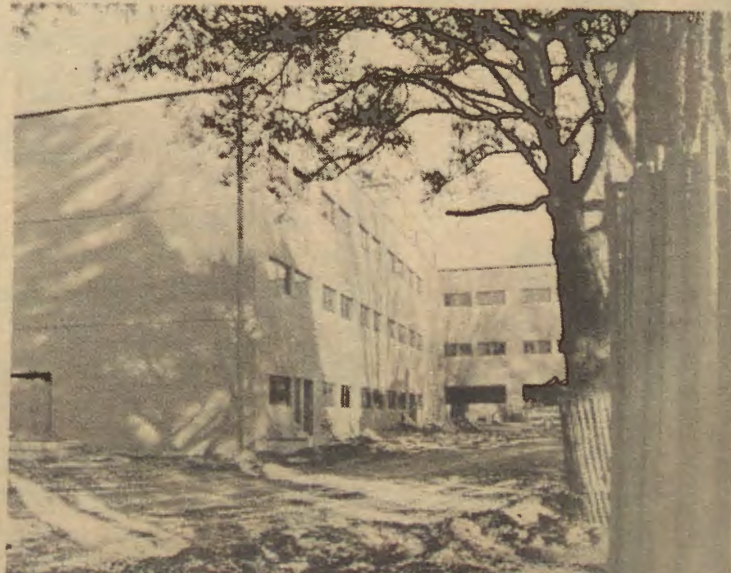
The new Fine Arts Building is under construction but materials being sprayed for fireproofing may be hazardous to your health. See story on pages 4 and 5. (Staff photo).
