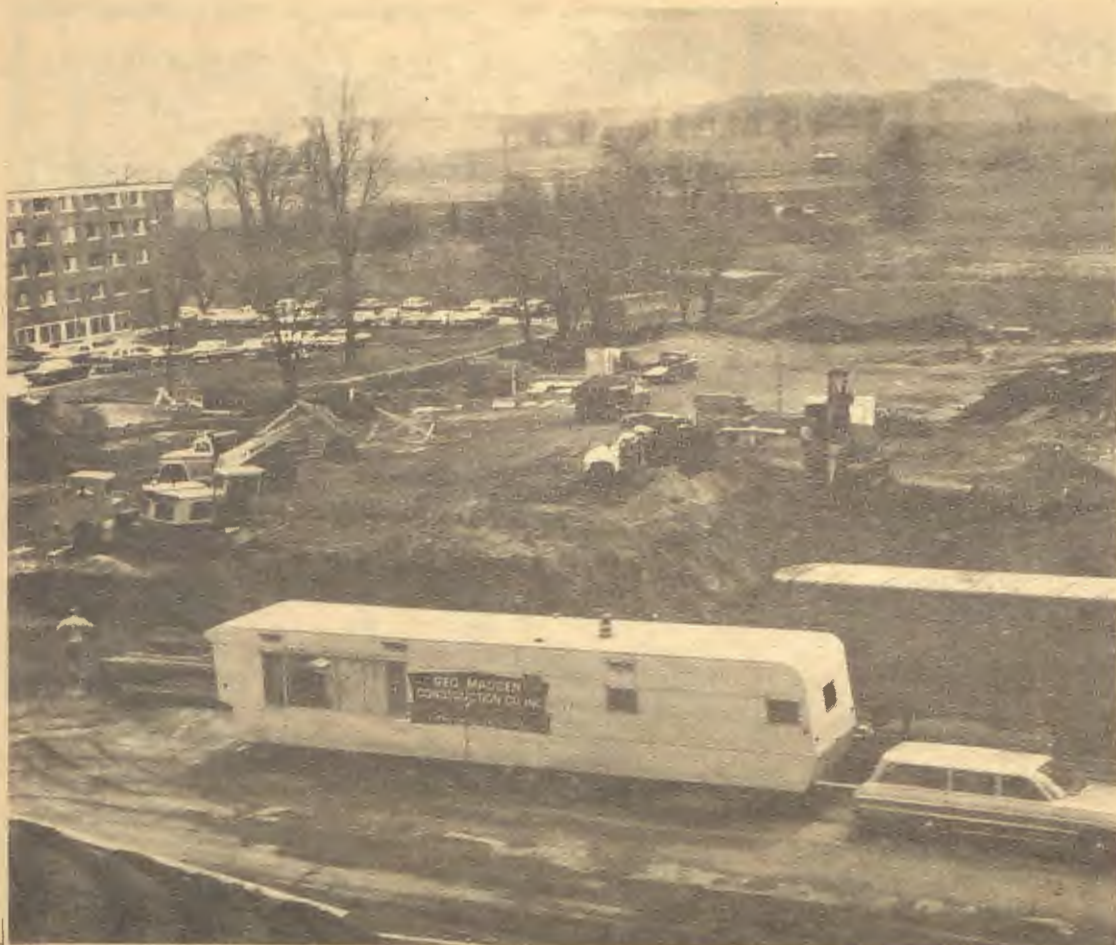
EXCAVATING FOR THE NEW SCIENCE BUILDING has begun. Construction crews leveled off the area behind the Student Center and are preparing to put in foundations.
